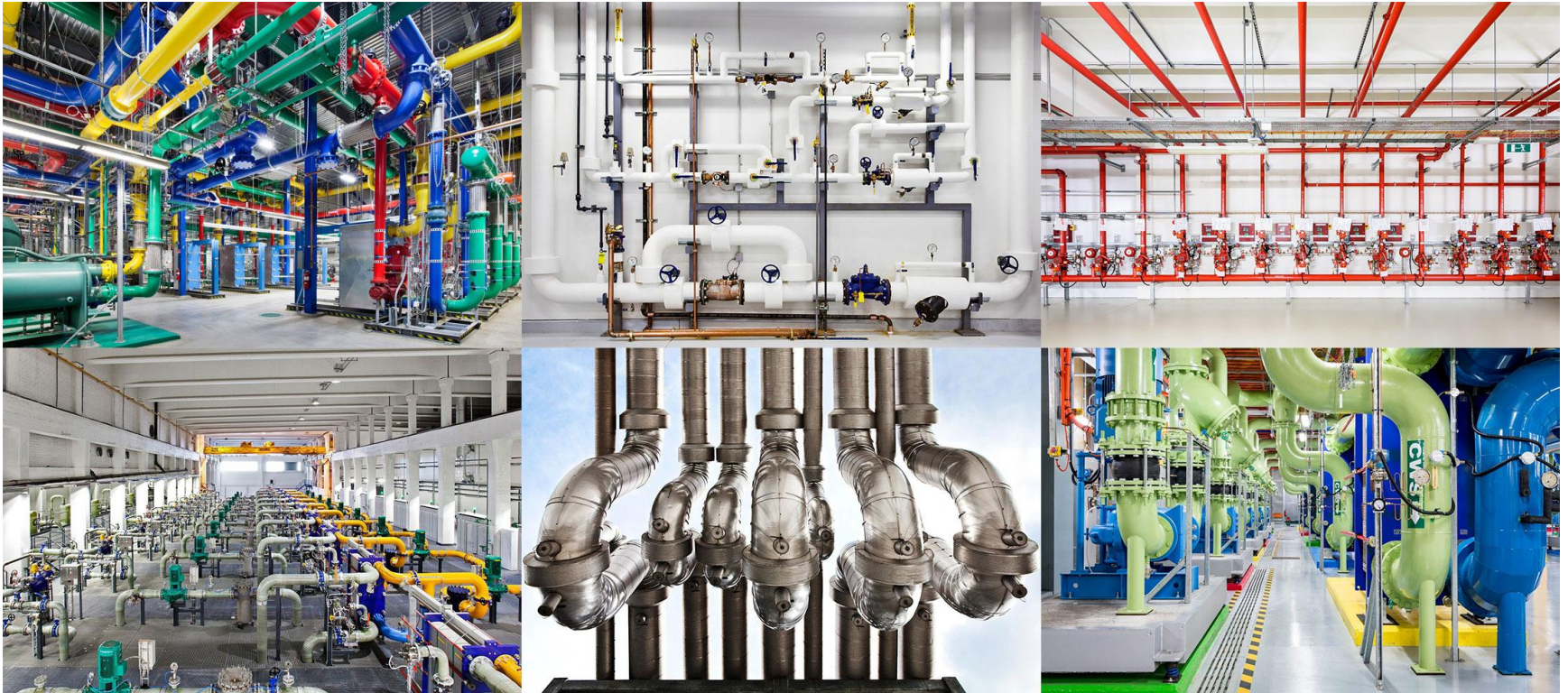
Large water pipes supporting the cooling system at a Google data center.
